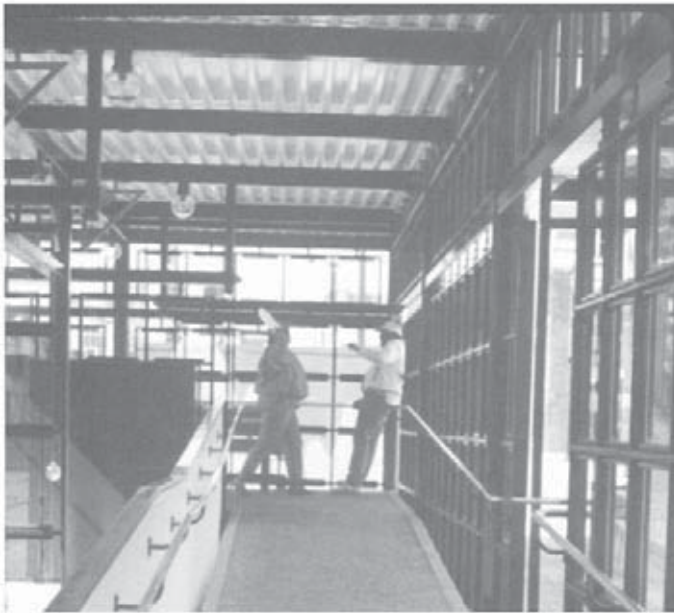
Figs. 6 and 7. Raised platforms for light rail work with ramps to provide access.
